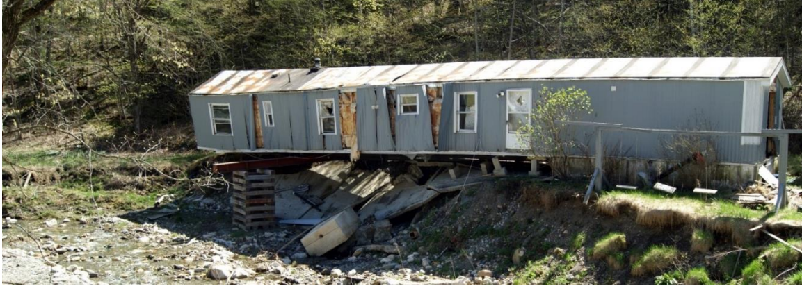
Structures built in floodplains like this one along the Danby-Pawlet Road are a risk for homeowners and the community at large. Floods can threaten to wash them downstream into bridges or other structures. Photo by Lori Fisher.
