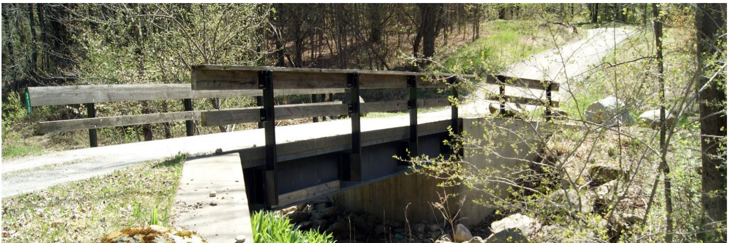
Of four stream crossings along North Road in Middletown Springs, this is the only one to have survived Irene. It was the only crossing built in consultation with a river scientist. Photo by Lori Fisher.
