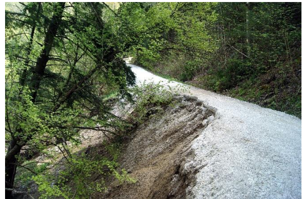
Upper Cold River Road in Shrewsbury washed away during Irene. Continued water seepage from the nearby hillside poses a significant construction challenge for this dirt road. Photo by Lori Fisher.
