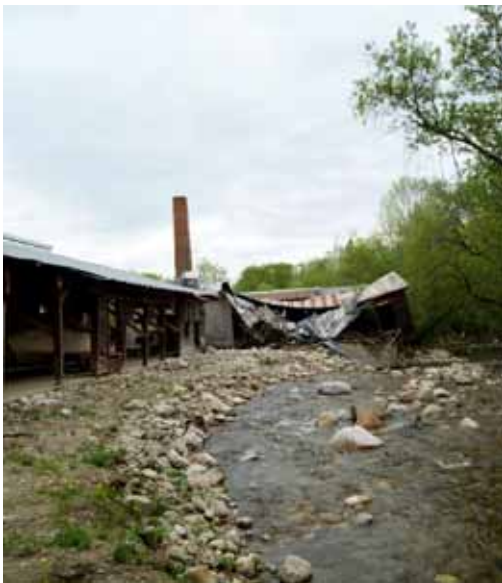
The former Vermont Tubbs furniture factory in Forestdale. The factory was destroyed when the Neshobe River escaped a berm on the left bank. Photo by Lori Fisher.
