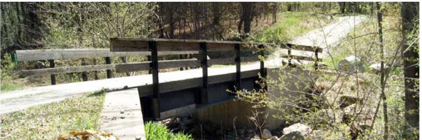
Of four stream crossings along North Road in Middletown Springs, this is the only one to have survived Irene. It was the only crossing built in consultation with a river scientist. Photo by Lori Fisher.
